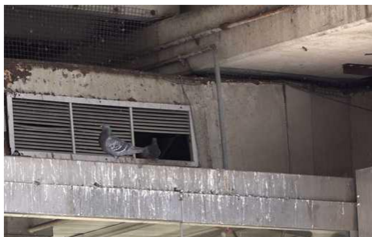
Figure 6: Image of Pigeons Nesting in HVAC Systems Along Perimeter of Alewife MBTA Parking Garage Station Complex [9]
