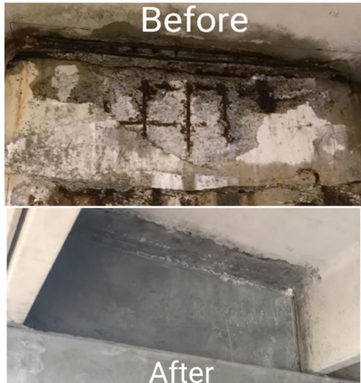
Figure 9: Image of Precast Beams Before and After Repairs at Alewife MBTA Parking Garage Station Complex [19]
