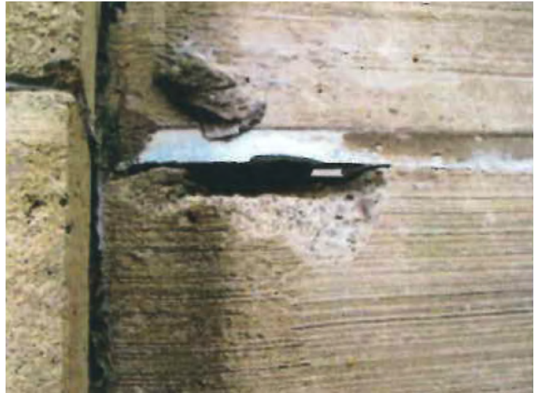
Figure 4: Image of Flange Joint Deterioration at Alewife MBTA Parking Garage Station Complex [3]
