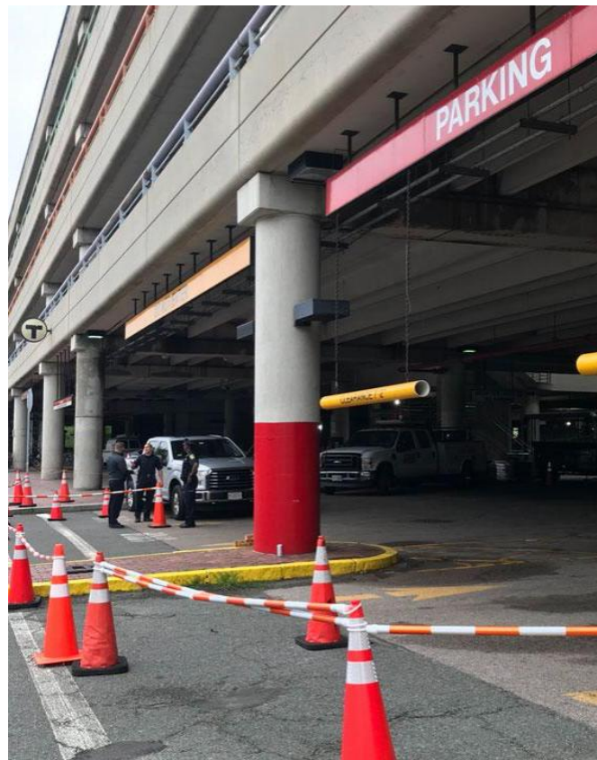
Figure 3: Image of Ongoing Construction and Rehabilitation Project Repairs at Alewife MBTA Parking Garage Station Complex [7]
